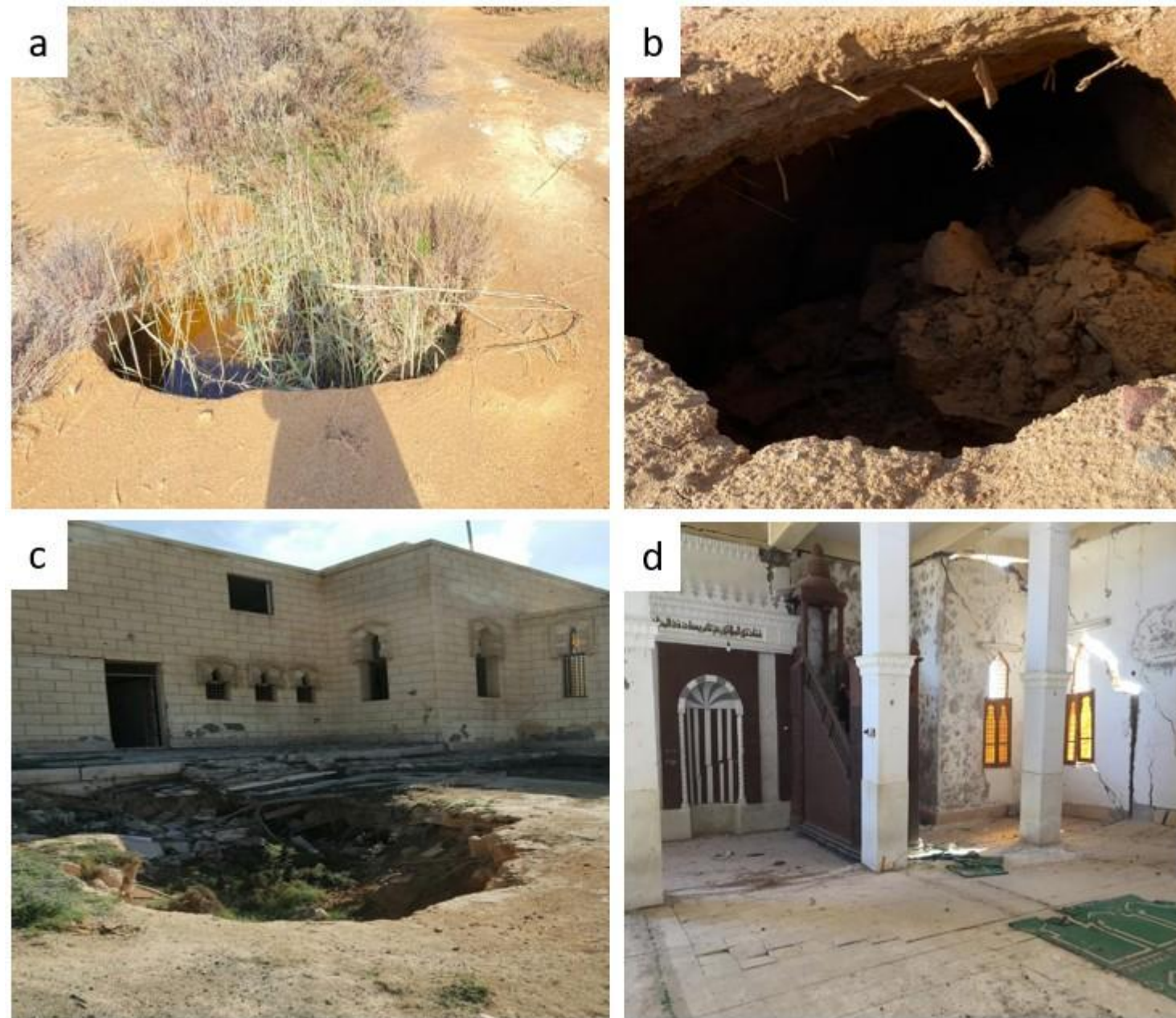
Figure 6. Manifestations of karst subsidence (a, b) sinkholes that formed due to karst, most of them filled with water. (C, d) Structural damage to buildings including tension cracks and subsurface voids
